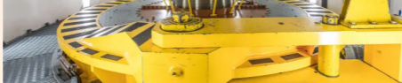
Snowy Hydro's Tumut 3 power station. When all six generators are pumping there is enough water flowing through the plant to fill an Olympic-sized swimming pool every two seconds
